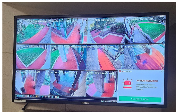
Courthouse Camera Monitors
