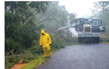
Responding to downed tree
