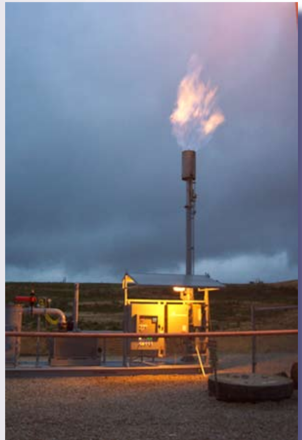
This methane gas flare is part of the new landfill gas collection and treatment system.
