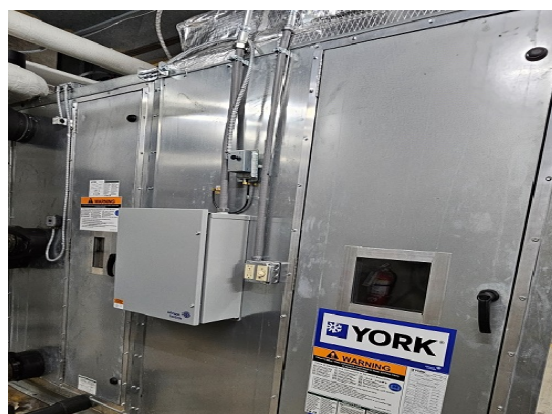
Building Mechanical Repairs and Improvements - Air Handler
