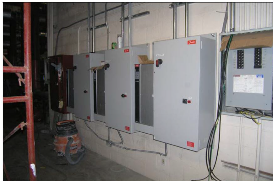
Architectural & Engineering Services- Electrical Panels
