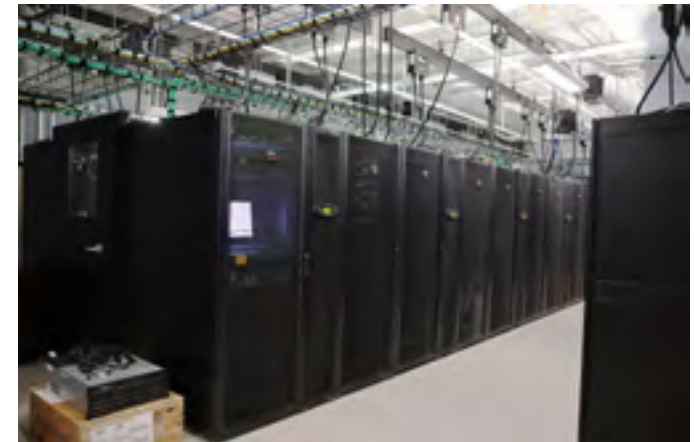
Public Safety Complex servers
