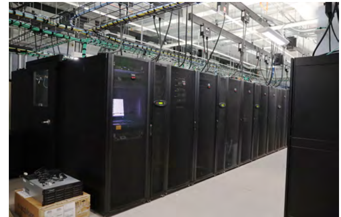
Public Safety Complex servers
