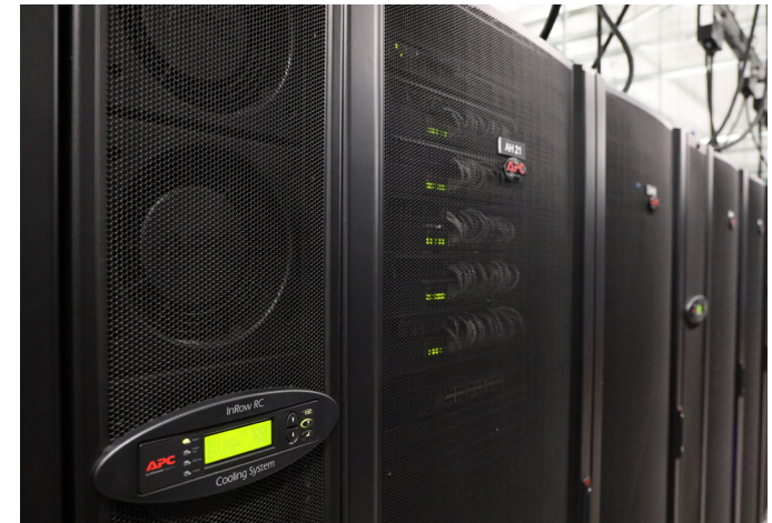
Public Safety Complex server room
