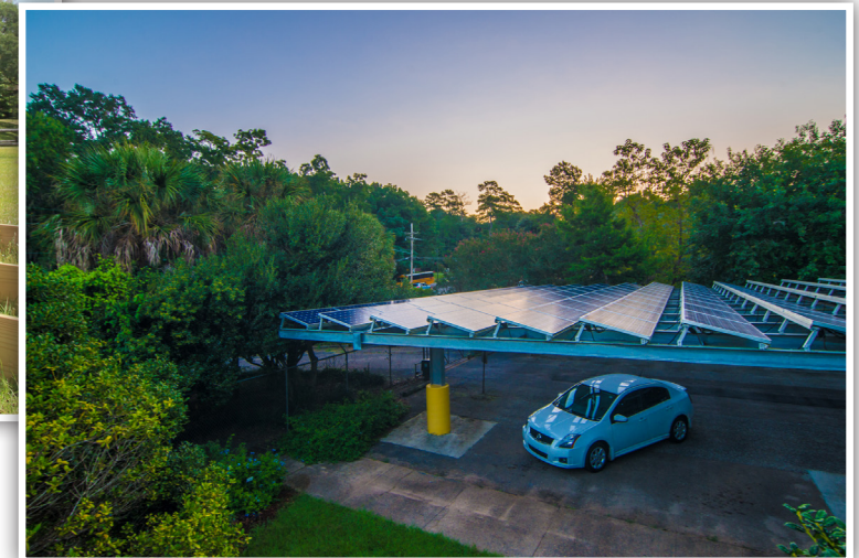
Leon County's Net-Zero Facility
