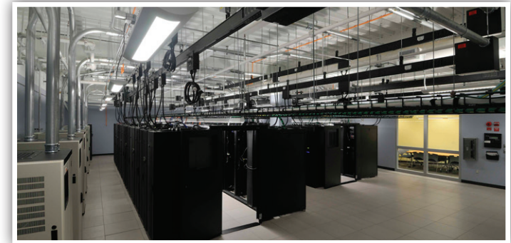
Public Safety Complex Data Center
